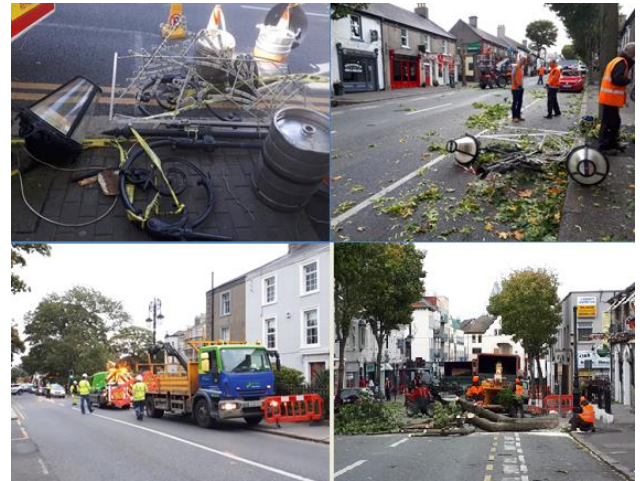
Damage and repair works resulting from Storm Ali
