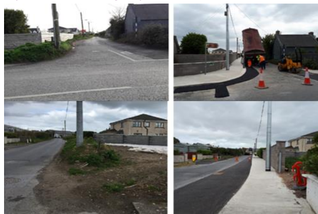
Works on a new footpath and road improvement scheme at Corrs Lane, Rush are nearing completion - before / after photographs
