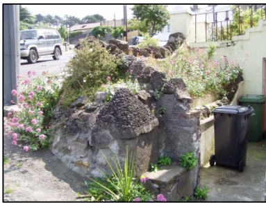
Fig. 6 Tufa capping to boundary wall
