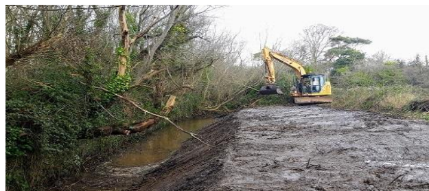
Drainage clearance works carried out of the River Pill in Newbridge Demesne.
