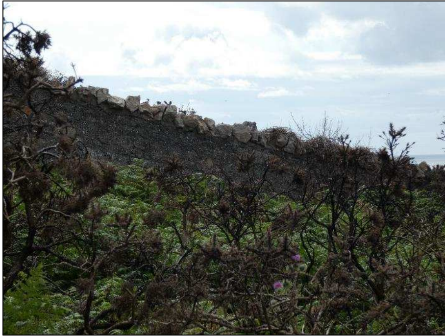
Plate 15. Close up of wall showing cement rendering
