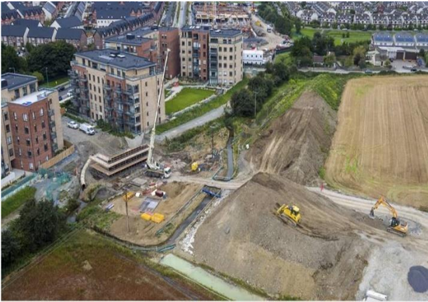
Stream diversion to allow construction of bridge abutments at FCC-DCC Administrative Boundary
