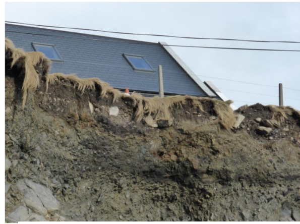
Figure 2-3 Shear eroded cliff face on the south coast of Inishbofin, Co. Galway. Extracted from RPS (2014)
