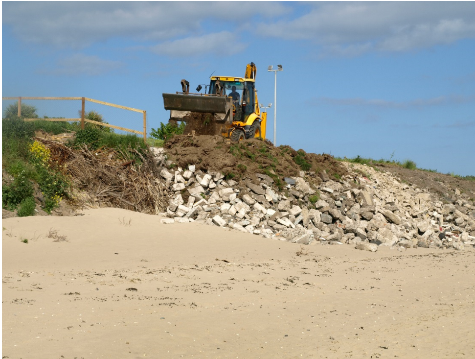
Figure 4-2 Landowners illegally dumping construction waste in an effort to protect their property.
