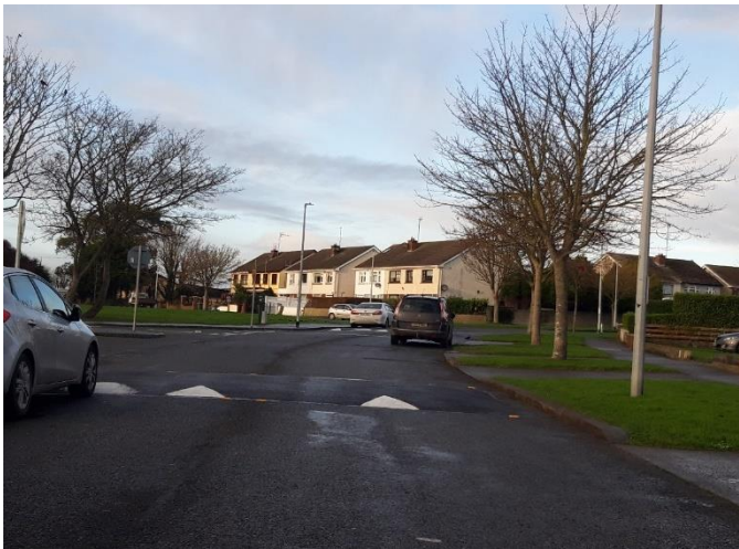
Newly installed Ramp - The Avenue, Rush, at St Catherine's National School with permanent Line marking and Studs in place.
