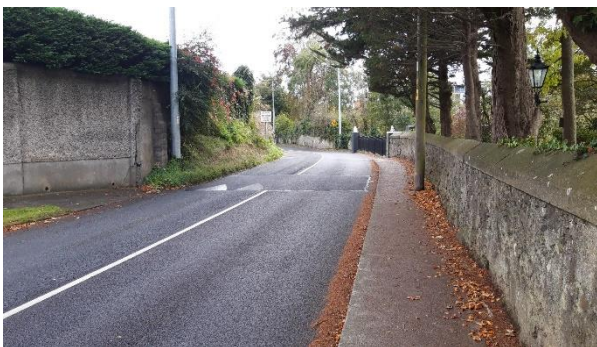
Swords, Brackenstown Road – Traffic calming ramps installed- permanent shark's teeth to be added
