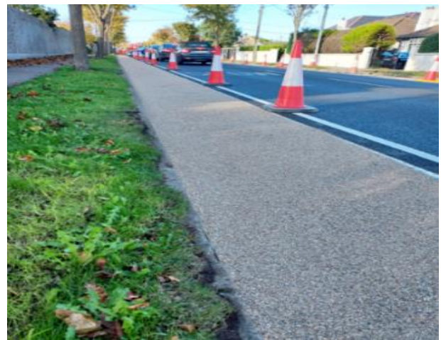
Baldoye – Howth Protected Cycle Lane Scheme: Night works and epoxy resin installation
