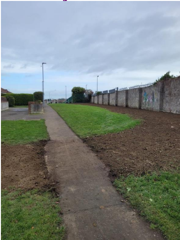
Castlegrange Estate - Levelling of grass area. Beech hedging also will be planted along entire length of wall. Further landscaping works planned in Autumn 2022 after phase one improvements are established.
