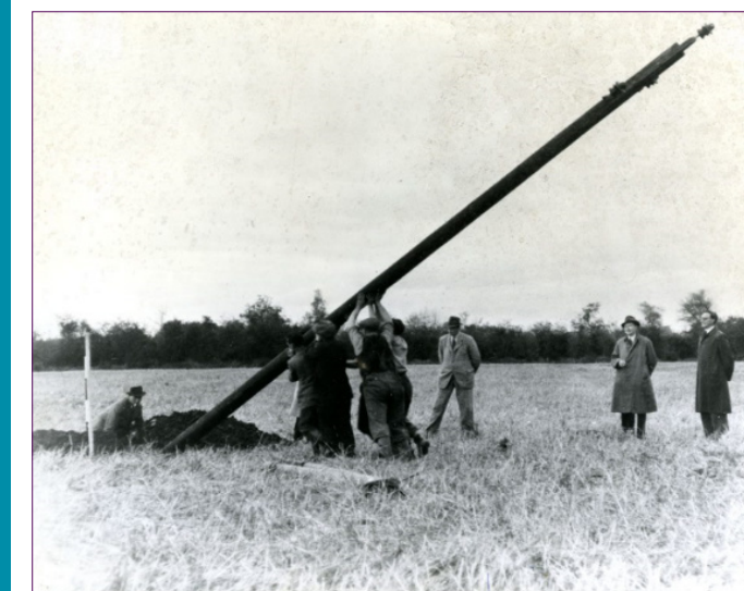
happen. Jan First pole at Kilsallaghan 5 November 1946 on to be remembered. Photo Credit: ESB Archives
