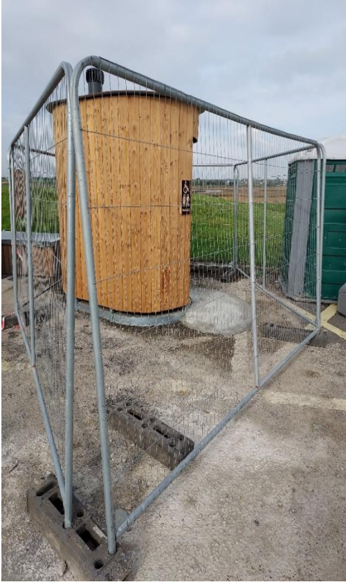
Portmarnock Beach car park (Strandmill) new replacement toilet is ready for ground installation.
