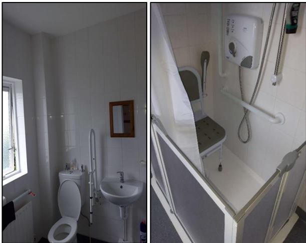
Level Access Shower and grab rails installed at Fingal dwelling under DPG Scheme
