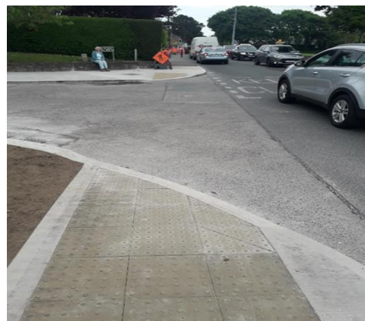
On site assistance provided to Road maintenance section in providing for new kerbing and tactile layout at the junction of the Hill Drive and Drumnigh Road (R124)
