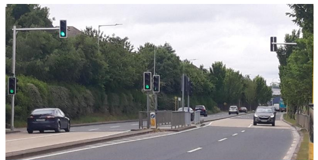
Holywell R125 – Signals Upgrade – New Outreach Signal Poles for improved visibility for motorists
