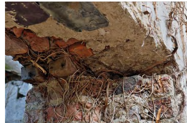
PIC. 17; LINTOL MISSING (OPE; VESTRY TO NAVE).
