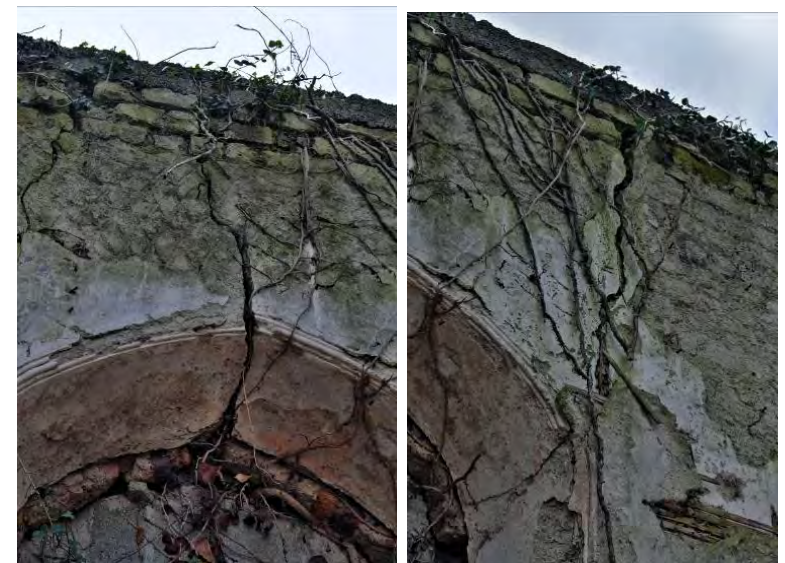
PICS 11 & 12; CRACKING IN MASONRY WALLS.
