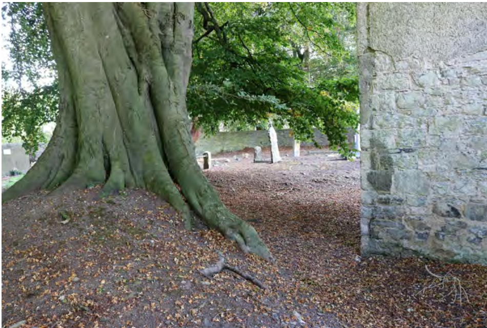
Figure 6: Base of tree beside north-eastern corner of church.
