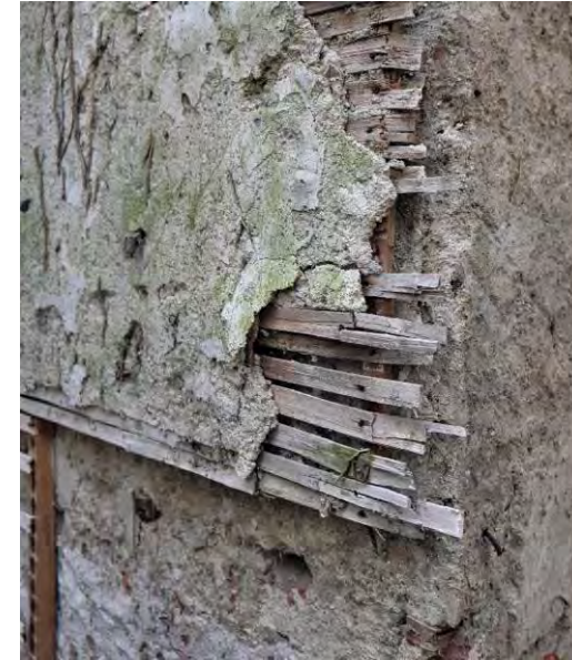
PIC.10; INTERNAL RENDER REMNANTS.
