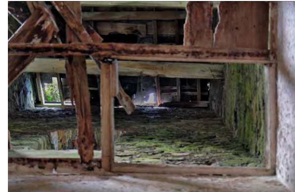
PIC. 16; (LOOKING THROUGH DECAYED FLOOR) LEAKING ROOF.
