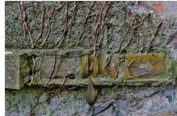
PIC.14; CEMENTITIOUS COATING TO BRICK SILL; IRON CRAMP.
