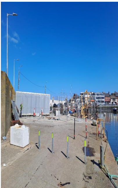
The sheet piles which form the berthing face of the bottom portion of Skerries Harbour have significant corrosion. A fence has been installed preventing access to the sheet piled section
