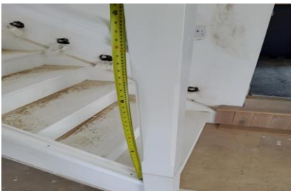
Checking banister height in a house in Loughshinny for compliance with Part K of the Building Regulations
