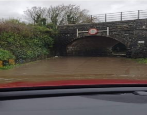
Barnageera Bridge flooded.
