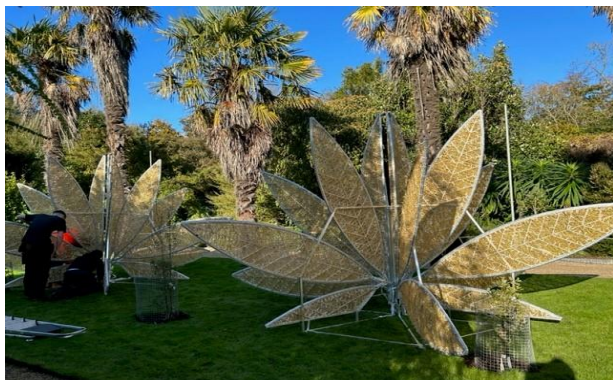
Work ongoing installing light features in Australian garden, Walled Garden Malahide Demesne
