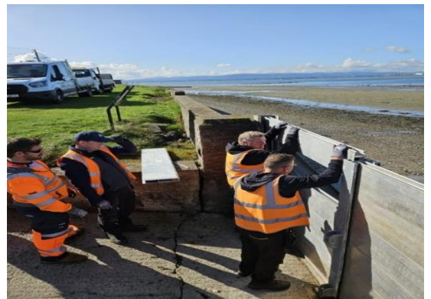
Flood Preparation works: Installation of the sea defence barriers at Sutton Strand
