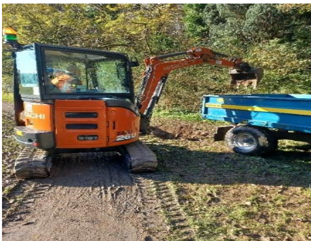
Remedial drainage works down at the dog run in the castle to alleviate pooling water.
