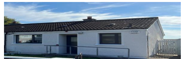
Post works – Strandmill Estate, Portmarnock (external wall insulation, new windows and doors)
