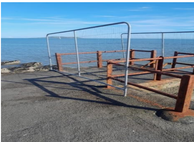
High Rock, Coast Road: During the rough seas and winds of Storm Babet, the ladder broke off. The location was secured by the crew preventing access to swimmers. New Ladder currently being fabricated and galvanised. Ladder to be installed very shortly.
