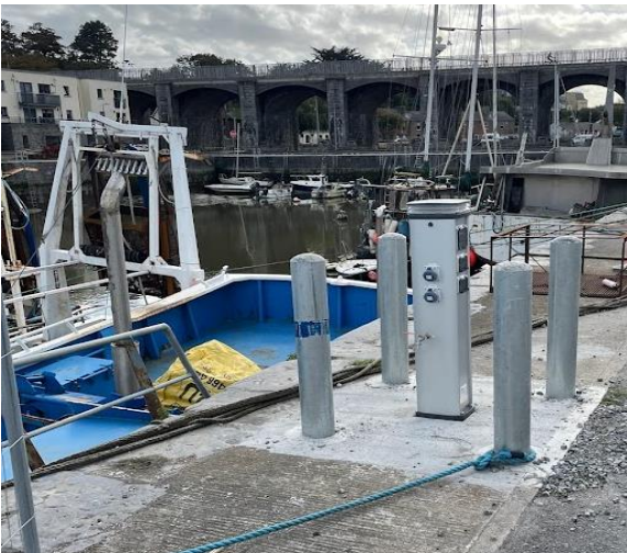
New Service Pedestals along West Pier, Balbriggan Harbour
