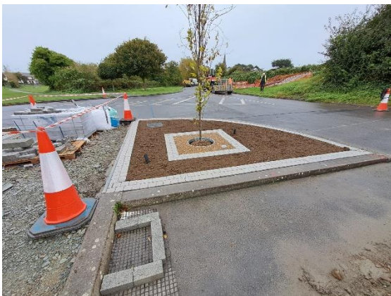
Newly installed Constructed Tree Pits and central median walkway to improve pedestrian accessibility from Skerries Mills car park into Skerries Mill
