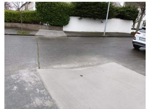
Meadowbrook Park- Baldoyle, Dishing of footpath to improve mobility for wheelchair users and mobility scooters.
