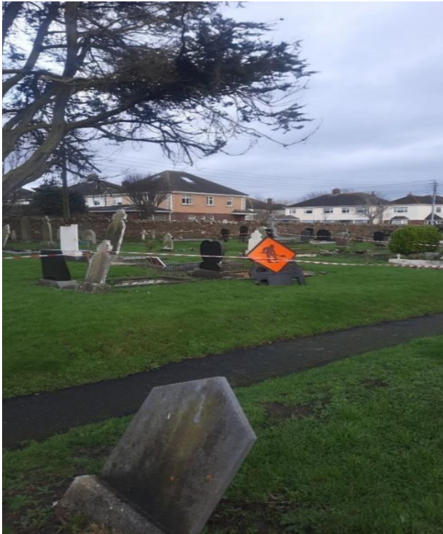
Kilbarrack burial grounds removal of dangerous tree from storm damage complete
