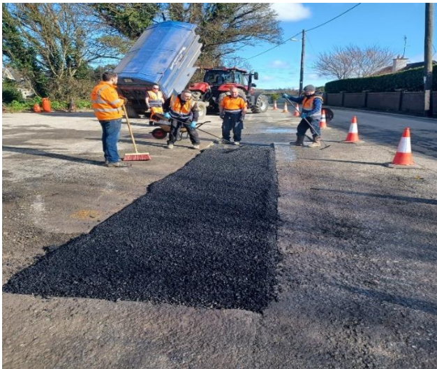
Wearing course being laid as part of deep patching repairs by FCC Crews on Kinsealy Lane
