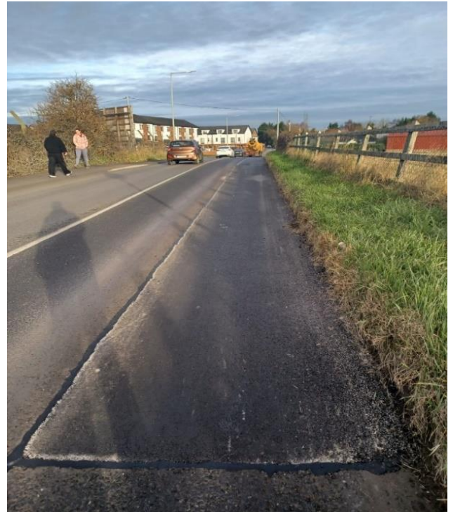
Substantial patching repairs on Feltrim Rd carried out FCC Operations Road Crews
