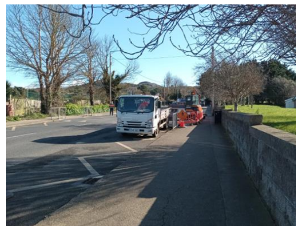
POW 2024 – Commencement of conversion of an uncontrolled crossing to a Zebra crossing by St Fintan’s National School on Carrickbrack Road-Sutton
