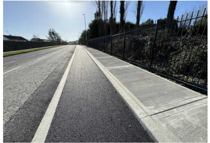
Works progressing on Harry Reynolds Road just north of Fingal Bay Business Park with Footpath and cycle track installed recently.
