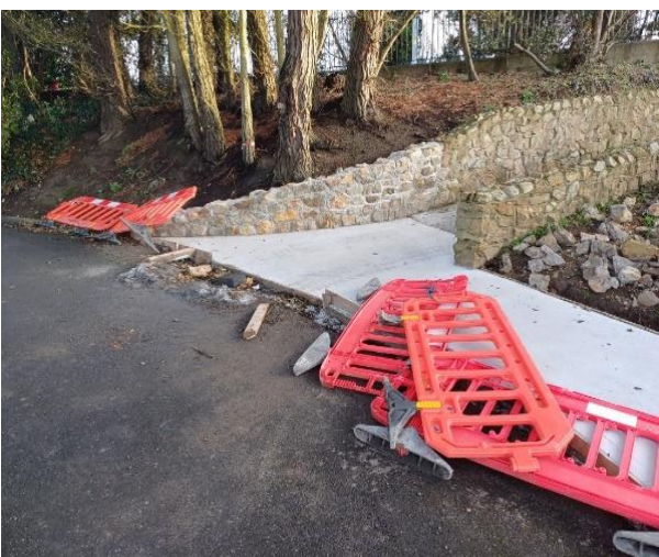
Replacement concrete aprons and stone wall repairs at St. Fintan's burial grounds on going.
