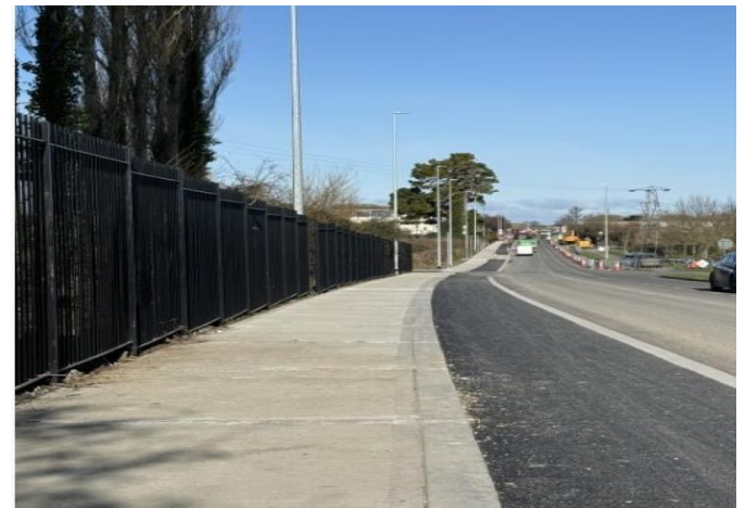
Works progressing on Harry Reynolds Road just north of Fingal Bay Business Park with Footpath and cycle track installed recently.
