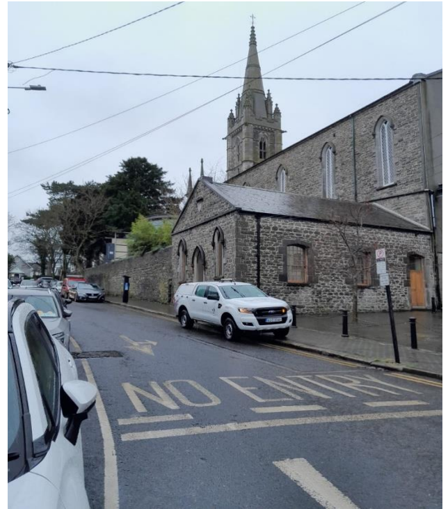
Power washing and cleaning at the square rear of Malahide church works completed.
