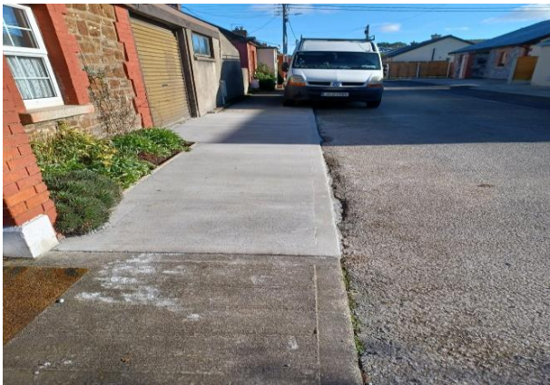
Replacement of Defective Footpaths in Bayside reported through the CRM system.
