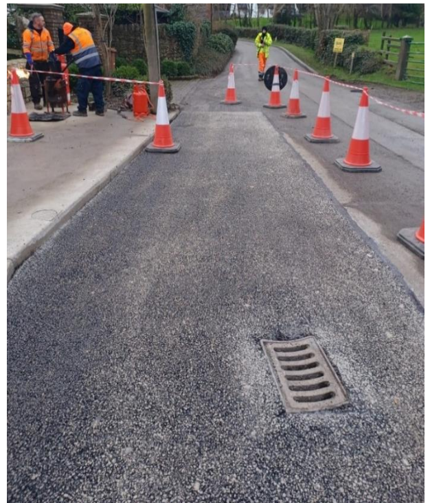
Substantial patching of Streamstown Lane carried out by FCC Operations Crews. Potholes reported through CRM system.
