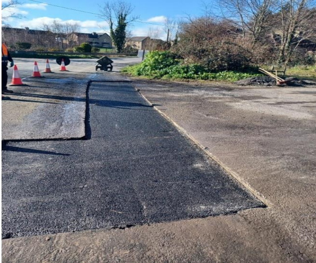
Substantial patching repairs carried out by Fingal County Council on Kinsealy Lane
