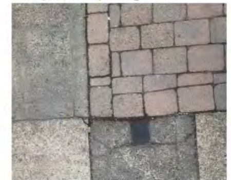
Poor and inconsistent paving materials
