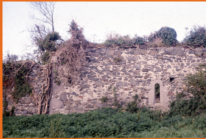
South wall of the fortified house prior to reconstruction. Paddy Healy Collection
